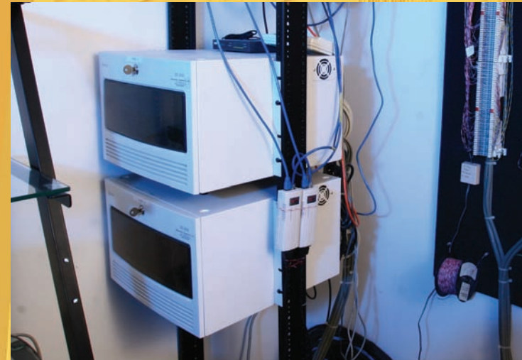
Our Servers are located in their own, locked-down, secure room.
